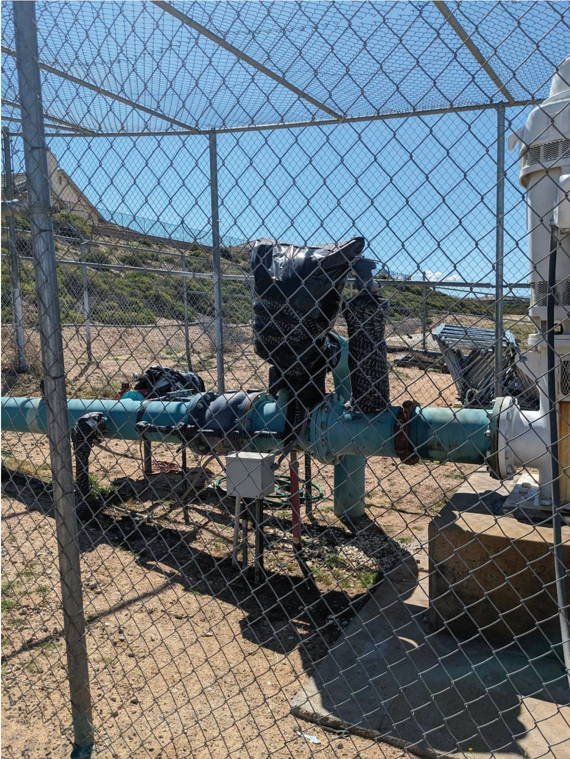
Figure 5. Well 34 with insulation on piping.
