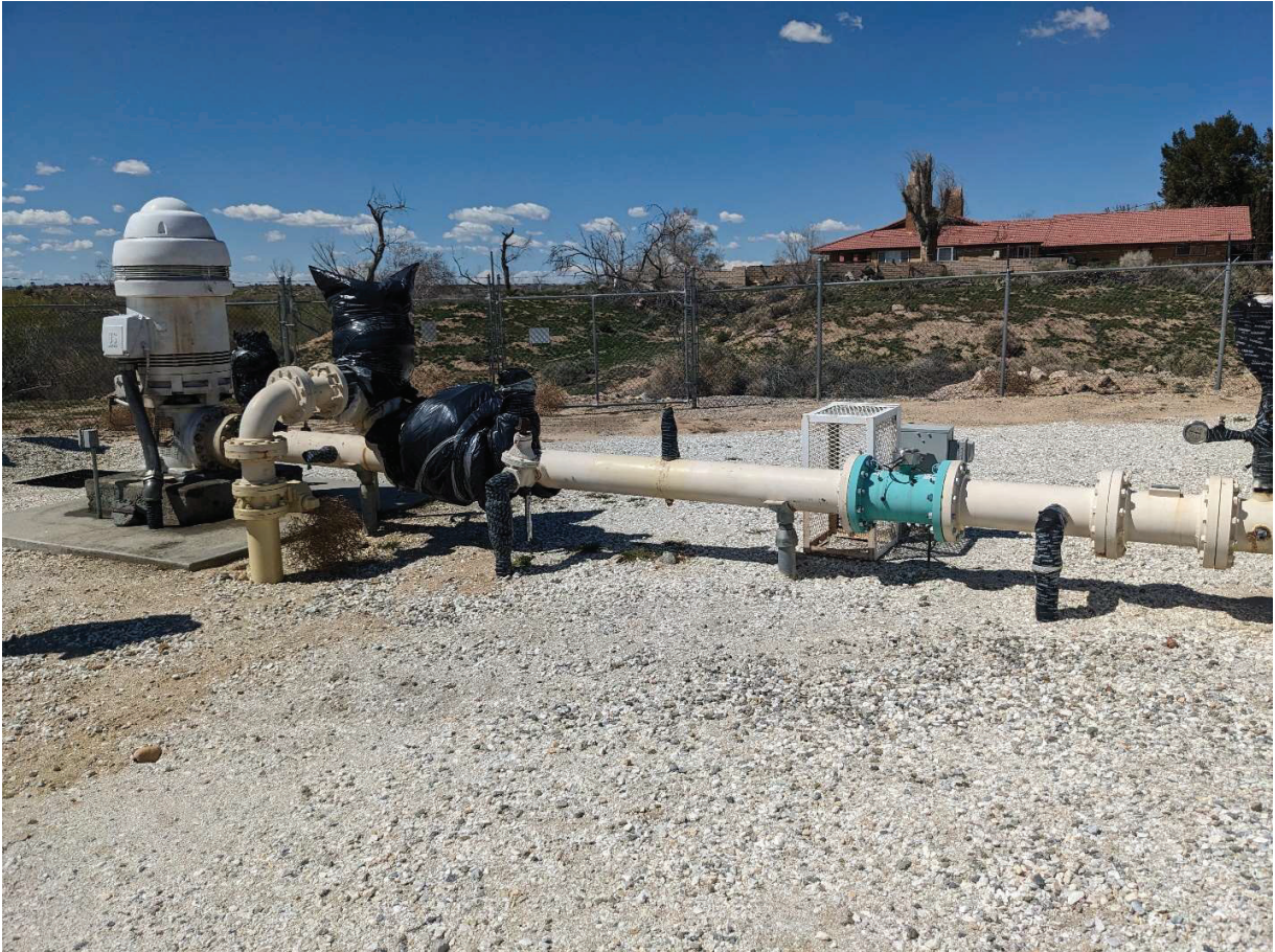
Figure 1. Well 18 with insulation on piping.
