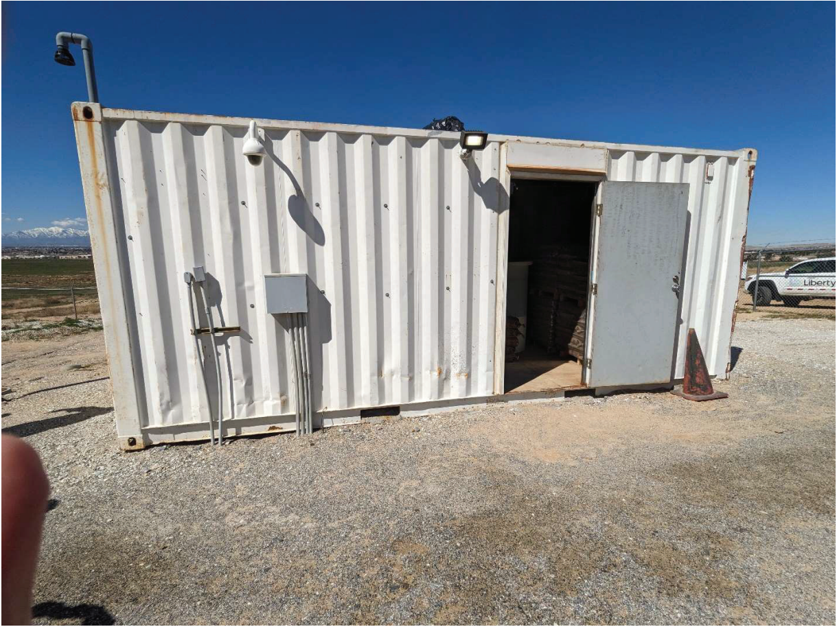
Figure 6. Disinfection Equipment Container for Well 34.
