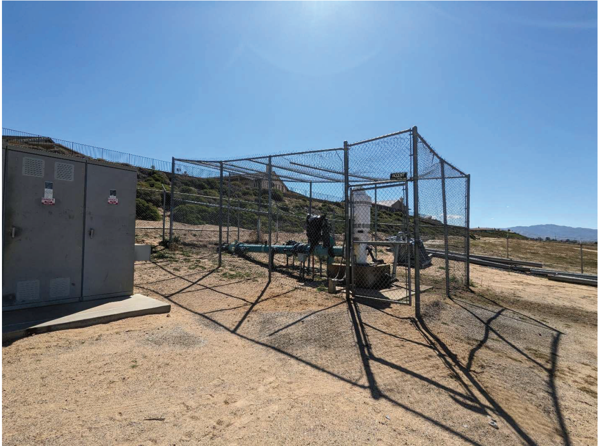
Figure 4. Well 34 with chain-link enclosure.
